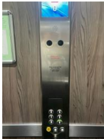
Lift controls and display.
